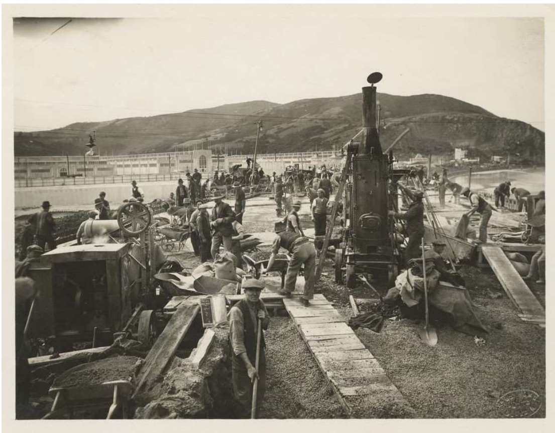
Building bridge over Water of Leith, Anzac Avenue, Dunedin, 1925. Charles Clark Armstrong, P2013-019-027. Photography Collection.
